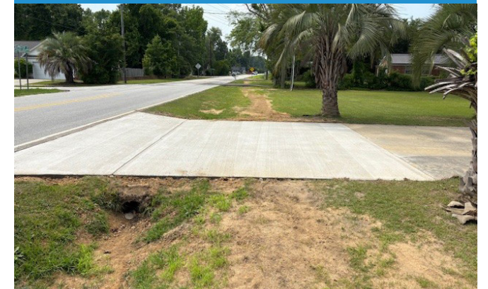
6 West Florence Distribution Upgrades
